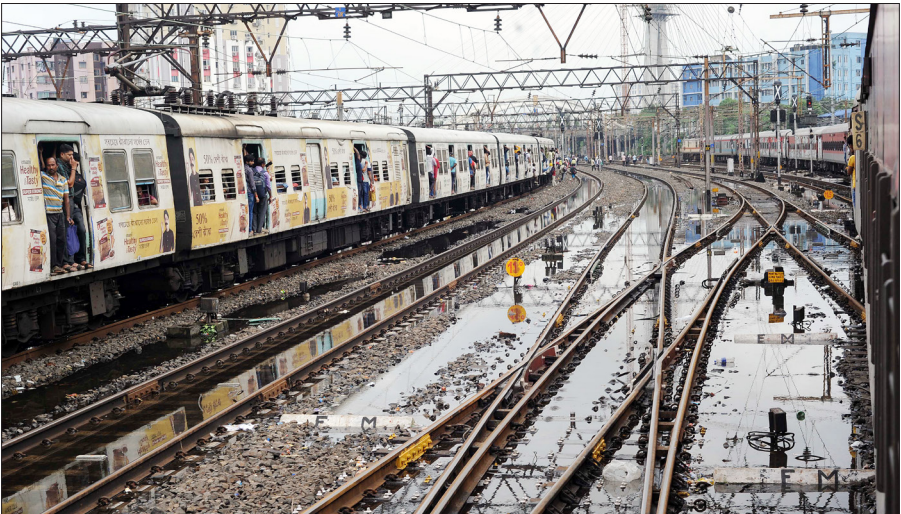
Howrah Car Shed Flooded Following Record-Breaking Rainfall in Kolkata on Tuesday.
