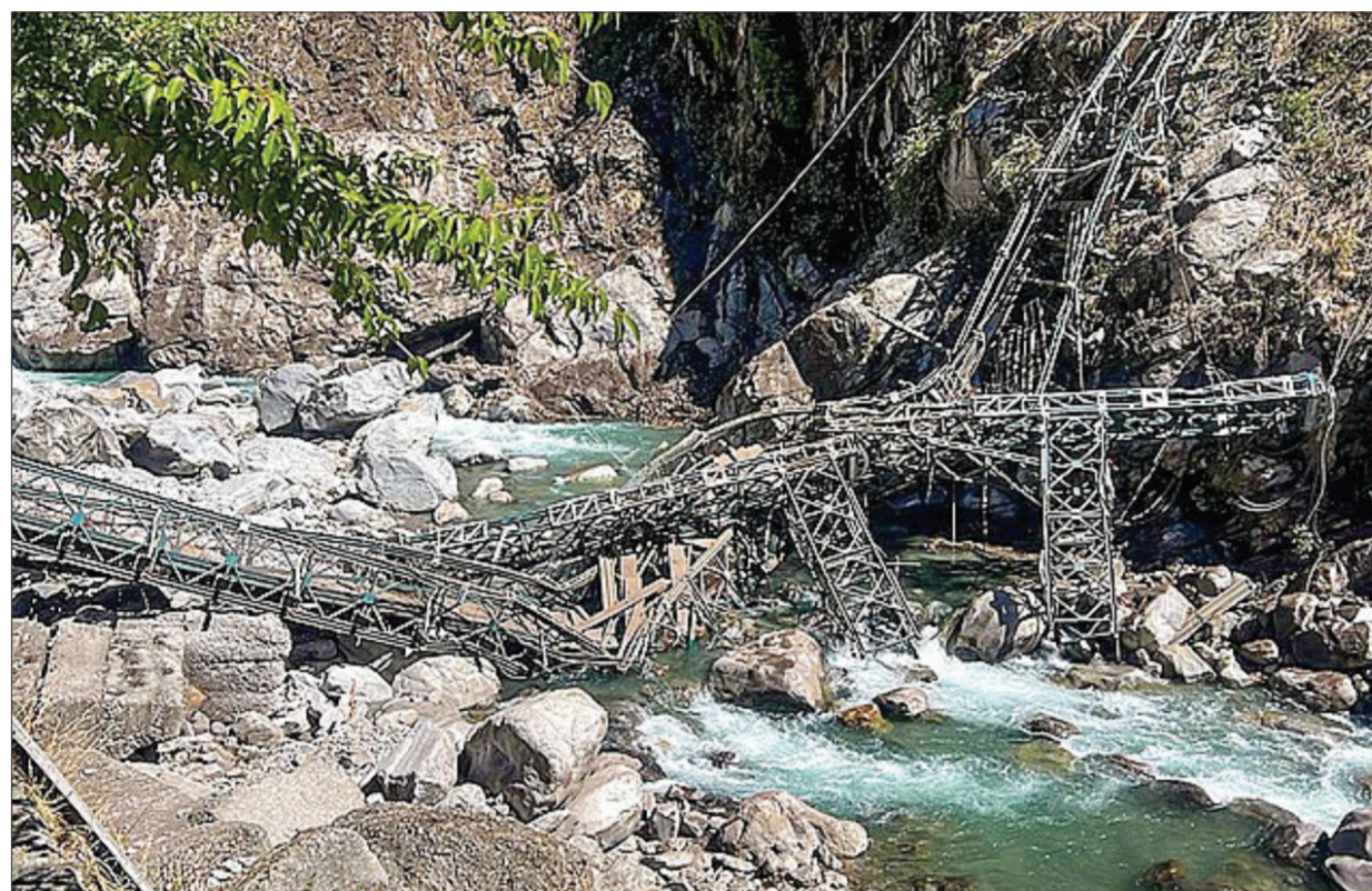
Damaged suspension motor bridge connecting Govindghat and Hemkund Sahib following a landslide, in Chamoli district.
