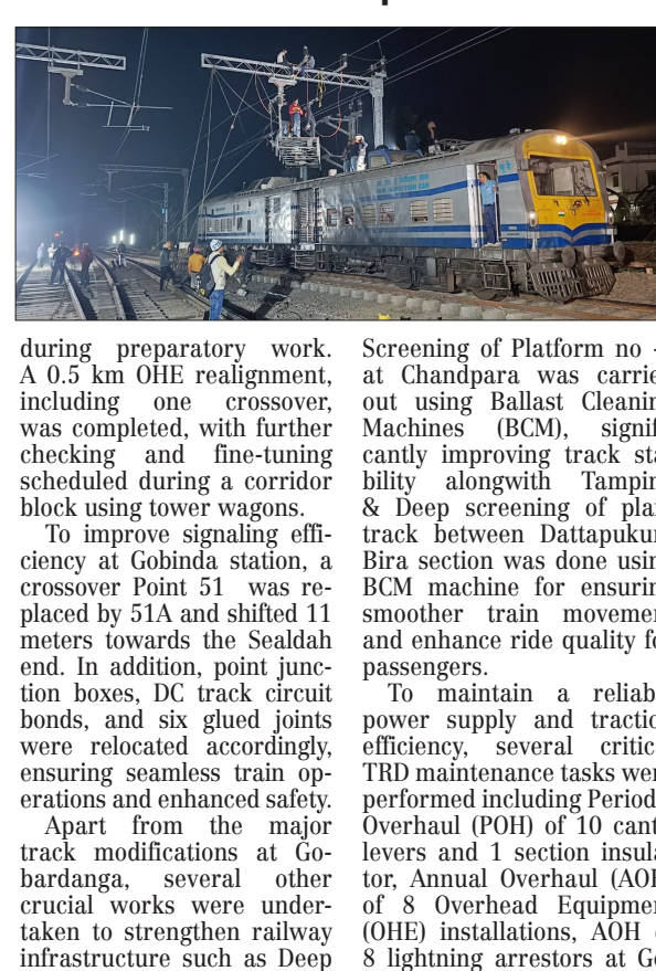
during preparatory work. A 0.5 km OHE realignment, including one crossover, was completed, with further checking and fine-tuning scheduled during a corridor block using tower wagons. To improve signaling efficiency at Gobinda station, a crossover Point 51 was replaced by 51A and shifted 11 meters towards the Sealdah end. In addition, point junction boxes, DC track circuit bonds, and six glued joints were relocated accordingly, ensuring seamless train operations and enhanced safety. Apart from the major track modifications at Gobardanga, several other crucial works were undertaken to strengthen railway infrastructure such as Deep
