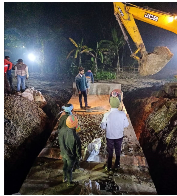
Advanced machinery was deployed for the execution of the work such as a 140 Ton Railway Crane, three Poelain machines, one JCB Breaker and one Hydra were used to facilitate the construction process. Additionally, several important maintenance works were carried out during the block. A total of 2400 Track
