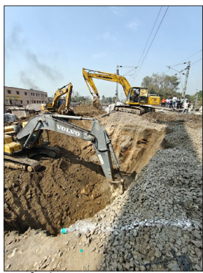
This method significantly enhances safety and strengthens railway infrastructure by ensuring superior earth retention, groundwater control, and excavation stability. It also minimizes risks such as track subsidence and soil displacement while improving worker safety and reducing disruptions to the surrounding area.
