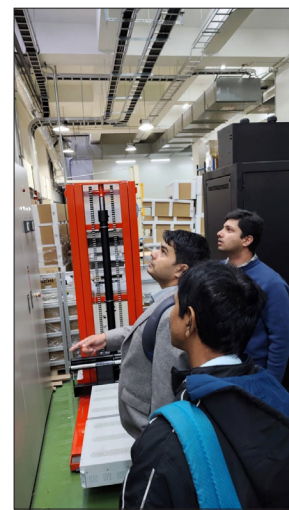
Delta Electronics Pvt. Ltd. on 04.05.2024 to install 4 MW BESS with 6.4 MWh Lithium Iron Phosphate (LFP) battery as energy storage element. Layout plan and manufacturing clearance was issued in the month of September-October 2024. With fast-track processing and manufacturing, the Advanced Chemistry Cell (ACC) Battery pack (LFP type) was ready for inspection in January 2025. Inspection was scheduled in the first week of February, 2025. A team consisting of Shri Abhishek Verma, Dy CEE/Maintenance/ Blue Line and Shri Uttam Kumar Bar, SSE/Masterda Surya Sen were deputed for inspection of battery pack at Taiwan manufacturing unit with approval of Railway Board. Inspection has been successful and dispatch clearance has been issued. It is expected that Battery pack will reach the installation site in the middle of March 2025. The system is expected
