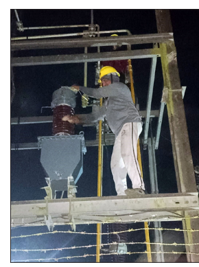
realignment encompassed 0.5 kilometers of wiring, including a crossover. Final checks and adjustments to the crossover alignment were conducted during a subsequent corridor block by replacing and shifting 11 meters towards the Sealdah (SDAH) end. This complex operation also included the relocation of point junction boxes, DC track circuit bonds, and six glued joints. This upgrade enhances the reliability and safety of point operations at this critical location.
